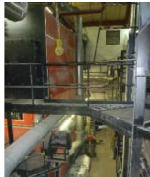
kotel na biomasu
